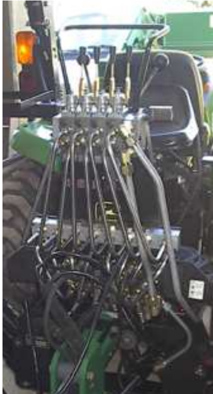
Figure 52: Haptic Backhoe hydraulic system
